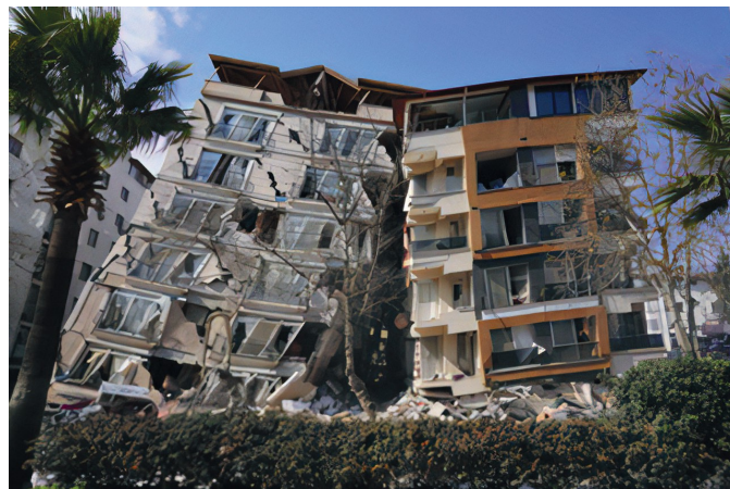
Figure 27: A picture of a collapsed building
