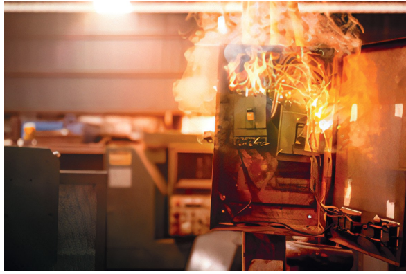
Figure 20: A picture of an electrical accident
