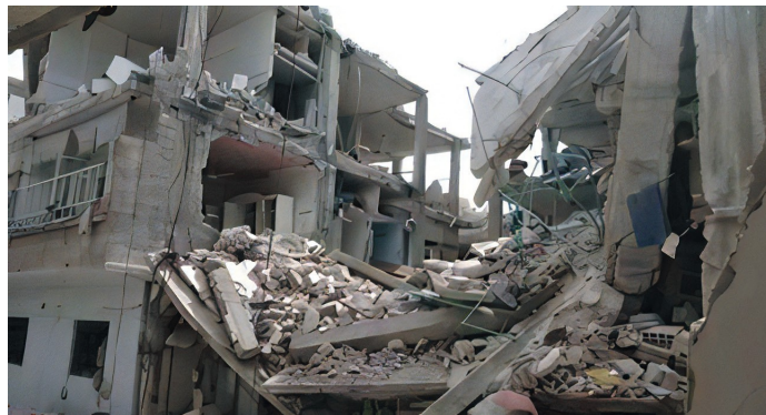
Figure 18: A picture of a structural failure
