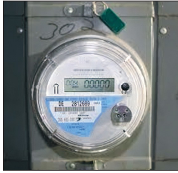
Figure 79: A picture of an Energy meter
