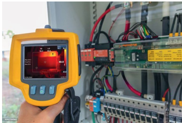
Figure 80: A picture of a Temperature Sensor
